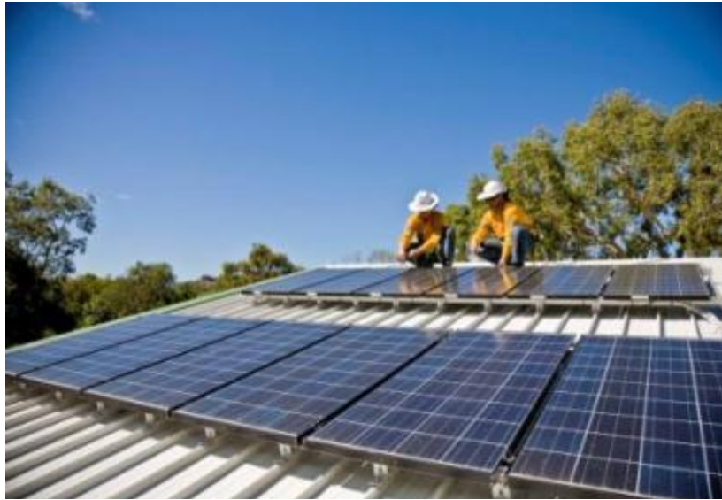
Flush mounted PV array on a Queensland School building (Photo: Ergon)
